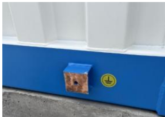
Figure 6 Partial view of grounding copper bar
